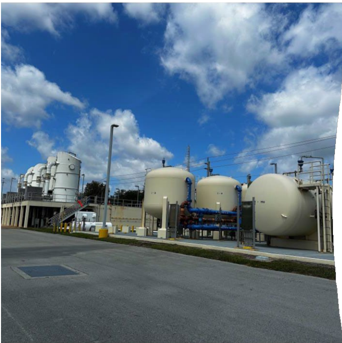
Picture 2: Ion Exchange & packed aeration towers
