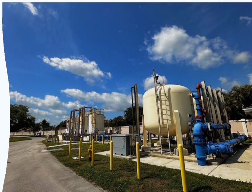
Picture 3: Ion exchange at the Southwest Water Plant
