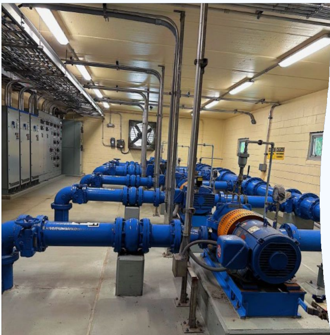
Picture 2: High service pumps
