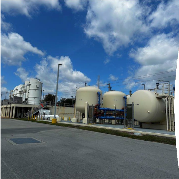
Picture 2: Ion Exchange & packed aeration towers
