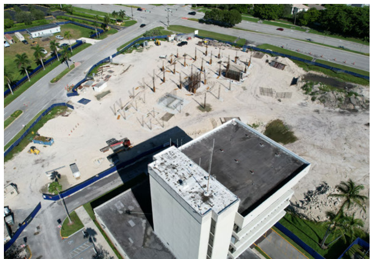
This recent drone image shows the current City Hall in the foreground, alongside the construction of the new City Hall structure.
