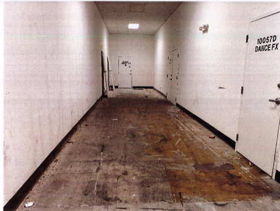
rear access to bay 10057B (formerly Sunshine City Trade) through internal hallway
